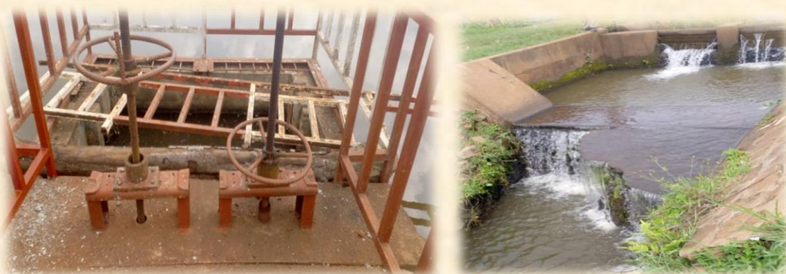
PHOTO 8: DEAD DAM GATES OR VANES THAT CONTROL WATER RELEASE AND DAMAGED SILL IN CYUNUZI
