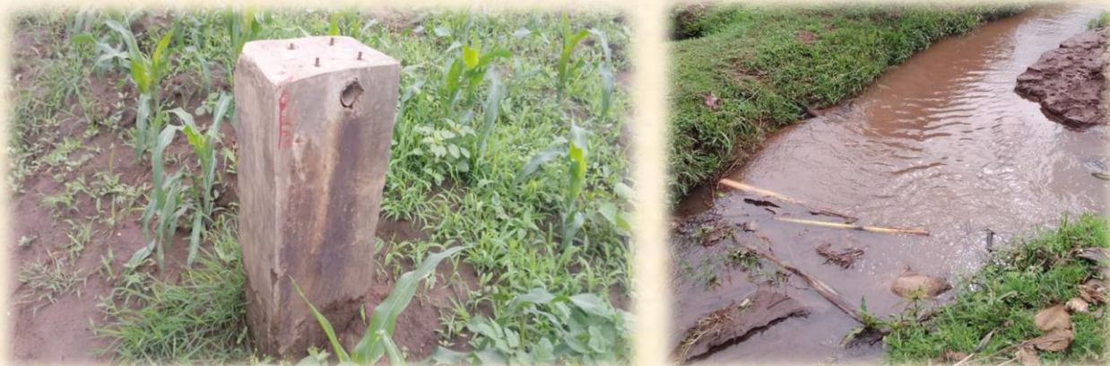
PHOTO 9: DAMAGED AND NON-FUNCTIONAL OUTLET IN KINONI AND DAMAGED SILL IN KINNYOGO
